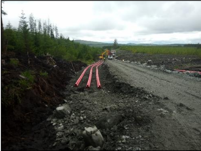
Plate 46 Looking northwest along ducting route between compound and substation
